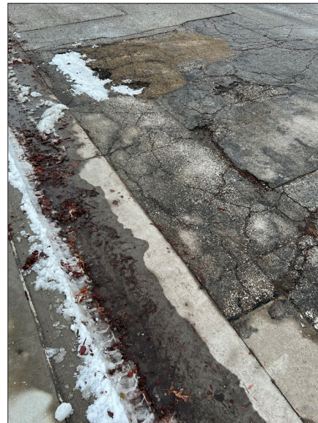
Figure 4.5 – Example of poor pavement conditions due to freeze/thaw cycle, Rock Island, Illinois
